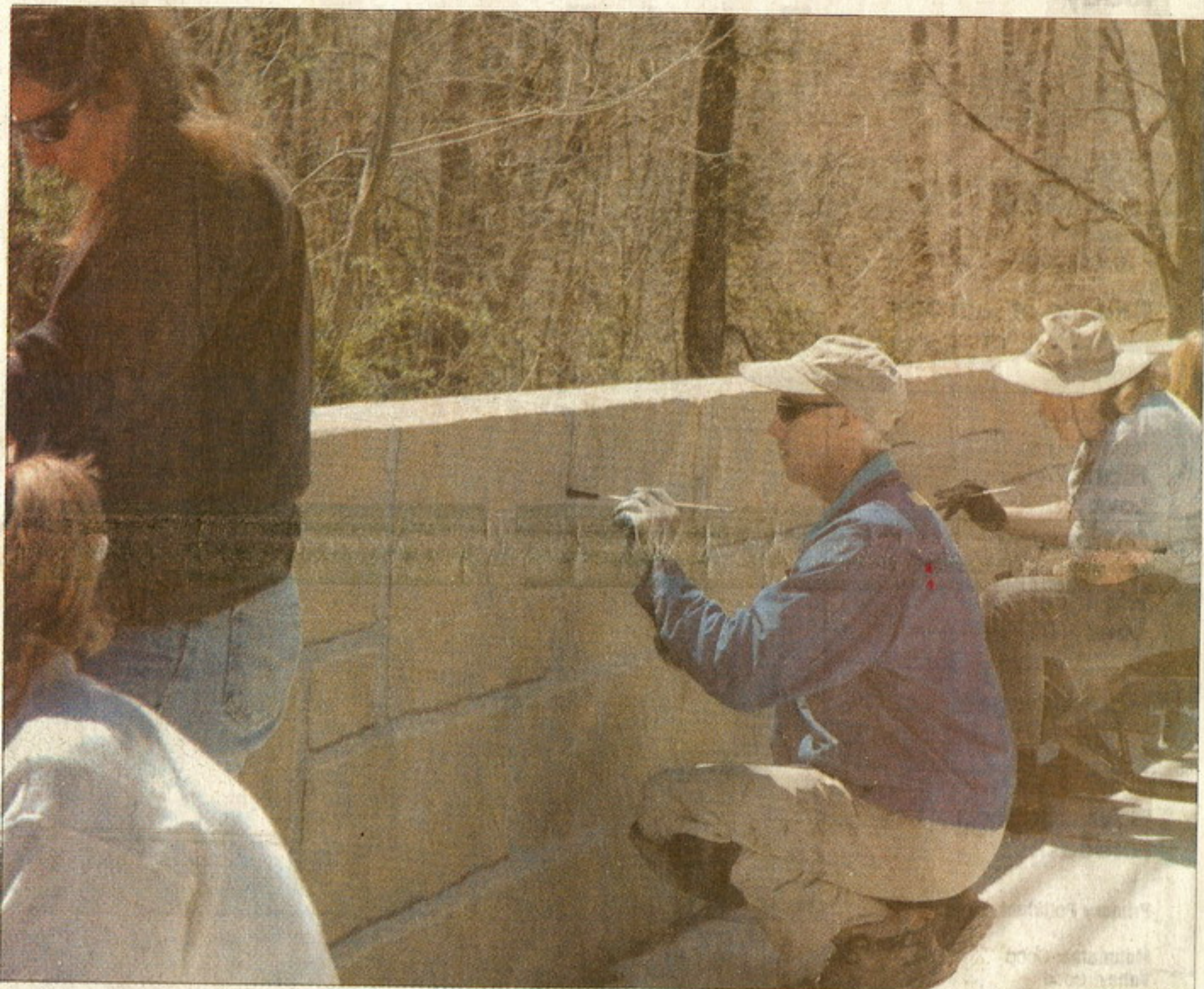
▲ Painters working for Michael Cooper of Murals & More began Monday to transform the concrete parapet walls along Highway 321 into "stone" walls. The large retaining walls on the opposite side of the road will receive a mottled paint effect that will help them blend into the background. For more on the project see story on page A5.
